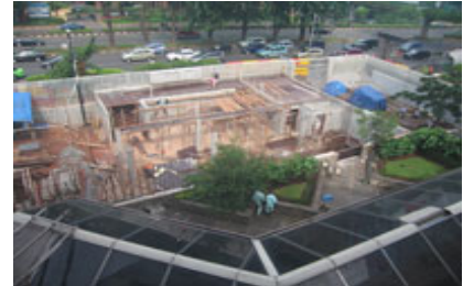
Repairs to the Australian embassy Jakarta and additional security works under construction following the terrorist bombing in September 2004
